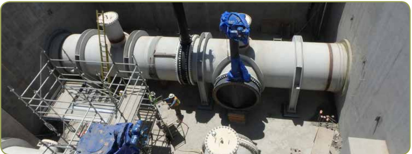
The flow-through diversion structure was successfully reconnected after the new outfall pipe was installed.
