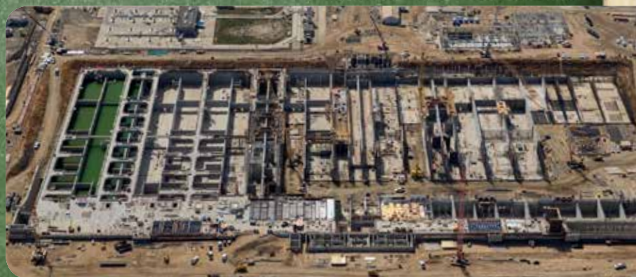
The BNR is the largest and most complex component of the EchoWater Project, with the basins alone taking up about 20 acres of land.
