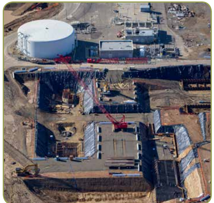
Crews excavated and winterized most of the TTF site to ensure heavy construction can proceed despite the winter rains.
